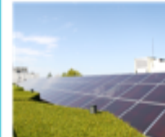
Roof top solar PV on Building 1
